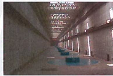
View of the completed Left Bank Powerhouse.
