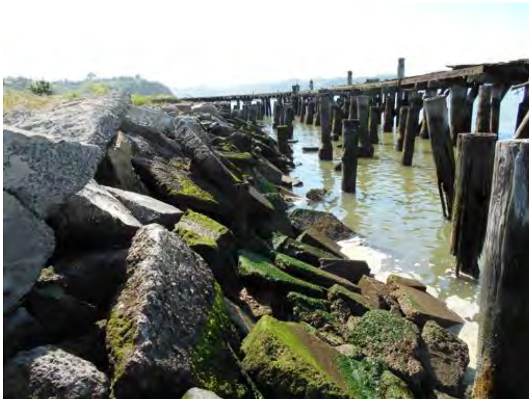
Figure 3-1 Survey Segment D, Concrete Slab Bulkhead. The light green algae is the filamentous form of Ulva spp. and the dark green is the leafy form of Ulva spp.
