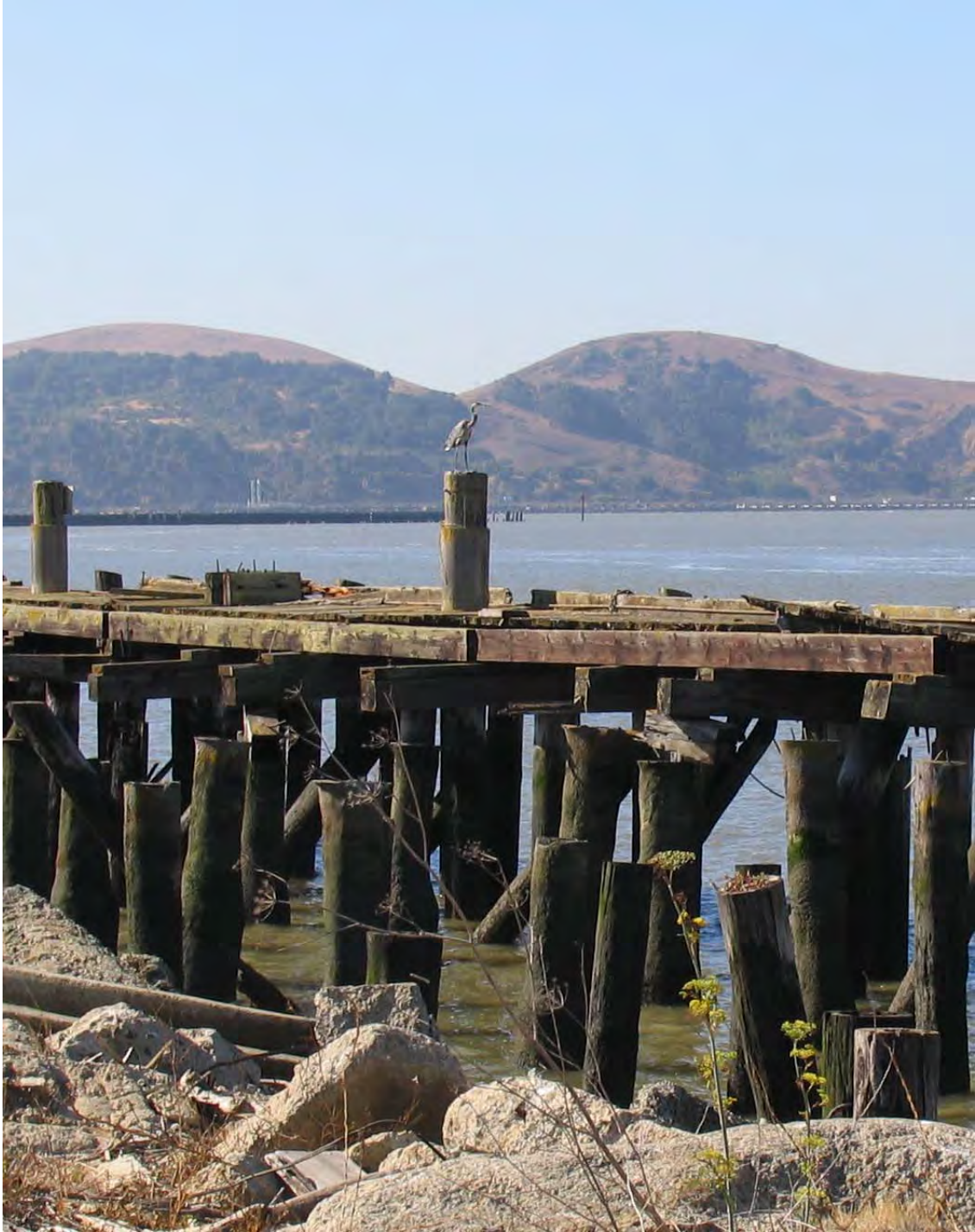
Representative example of piles and dock (with great heron). Carey & Co., Inc., 2007.
