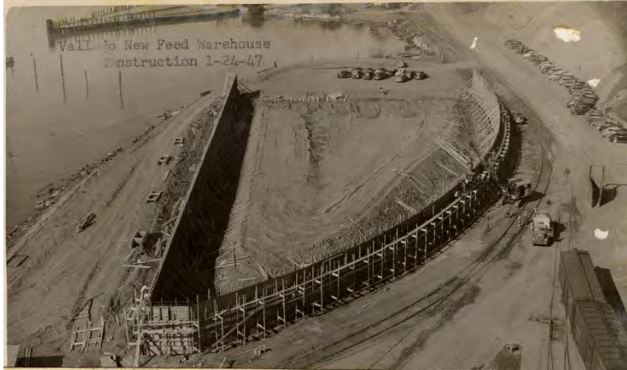
New feed warehouse, under construction, 1947. Courtesy of Floyd Miller and the Quarter Century Club, General Mills.
