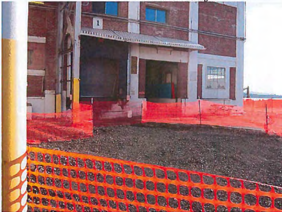
18. Former UST T-5 area, north Old Warehouse and Mill building, view to the southwest.
